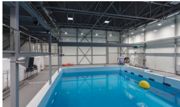
Constructing a new building for the Novikontas Maritime College in Riga, Latvia
