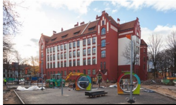
Improvement of the territory around the Fricis Brivzemnieks Primary School in Riga, Latvia
