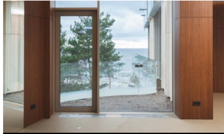
Construction of the Sea Breeze residential building at 2 Ērgļu Street in Jūrmala, Latvia
